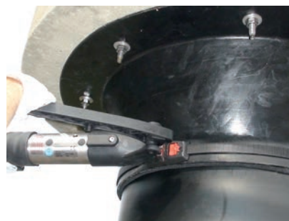
A 19mm band fixing is used to get a good seal over the existing SeaShield system
