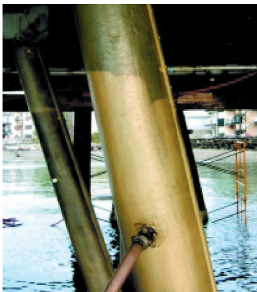
Pumping the SeaShield 550 Epoxy Grout. Note the visible rising level seen through the Form
