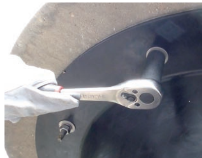
The Pile Cap is bolted to the underside of the jetty deck
