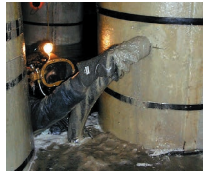
After fitting the Fiber-Forms the standard marine grout is injected by pump
