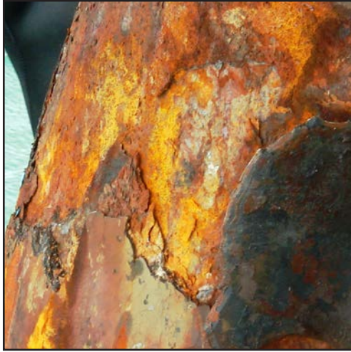
Example image of a pipe featuring loose corrosion that would require removal.
