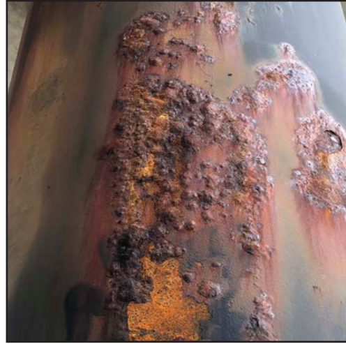
Example image of a pipe featuring a loosely adhering corrosion prevention coating that would require removal.
