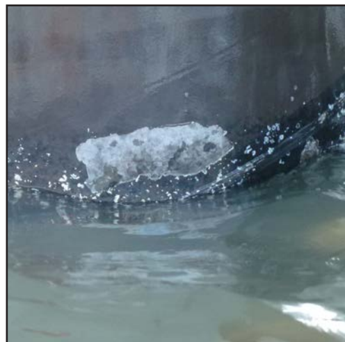
Example image of a pipe featuring acceptable levels of non-living, tightly adhering mineral deposits.
